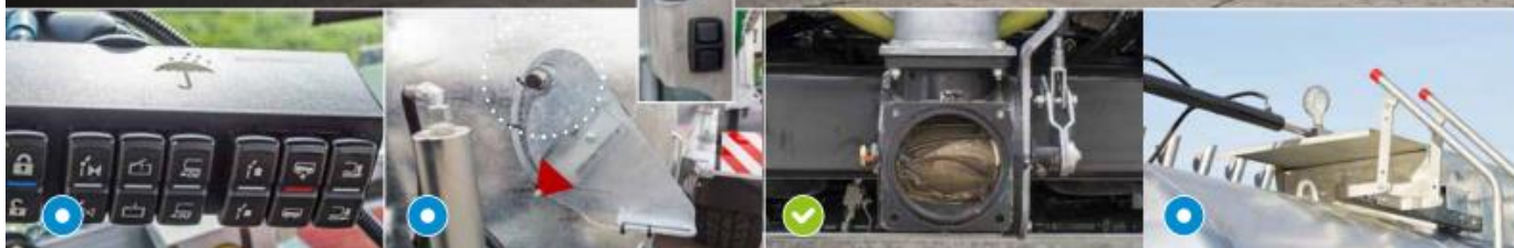
Control panel for tank + distributor
